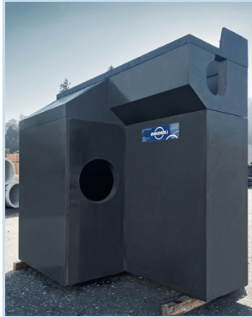
Siphon shaft enclosure in Schwamendingen. Inlet of slot drain (top right) and main drainage opening below.
