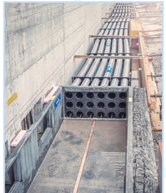
Cable shaft housing in Schwamendingen
